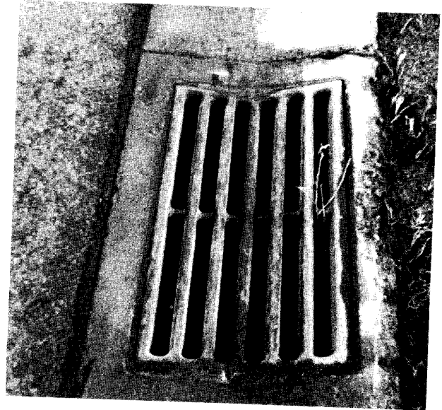
Figure 33. Drainage inlet designed for use with low mountable curb. Bars are oriented in the direction of flow.
