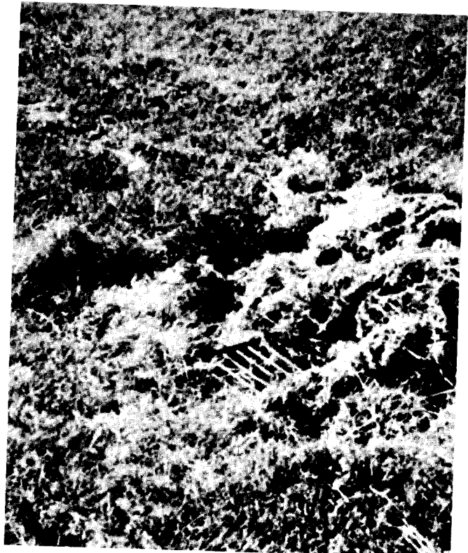
Figure 9. Capacity of drop inlet is threatened by debris and overgrowth.
