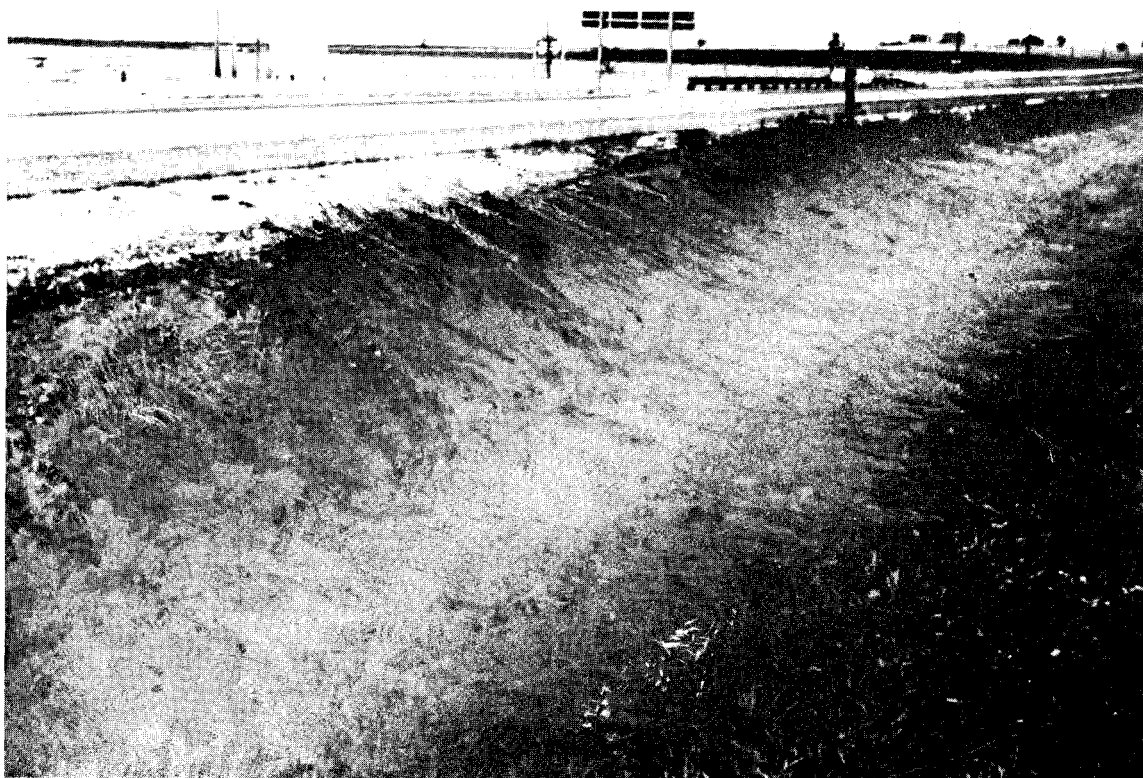
Figure 28. Closing of median crossover or drive entrance with guardrail barrier compounds hazards (top). Preferred solution would be to remove both the drainage structure and the guardrail and regrade the slope (bottom).
