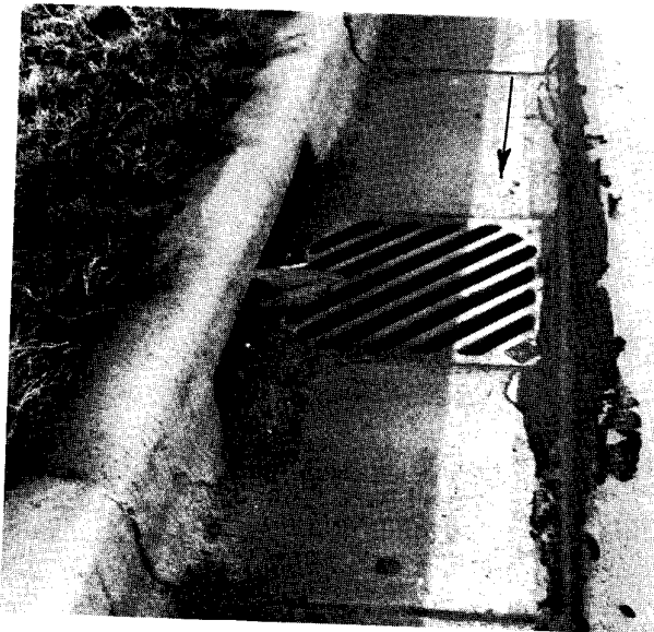
Figure 34. Drop inlet grate with bars positioned diagonally to deflect flow into curb inlet and to lessen hazard to narrow-tired vehicles.
